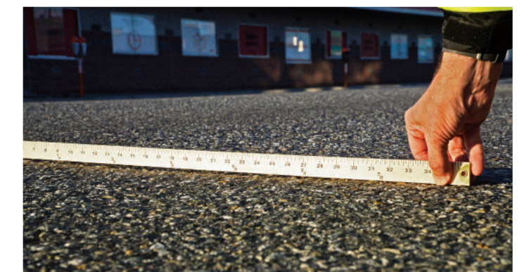
After four winter seasons (2015-2019), 200 block of E 5th Avenue with HiMA-modified PG 64-40 E binder shows minimal rutting
