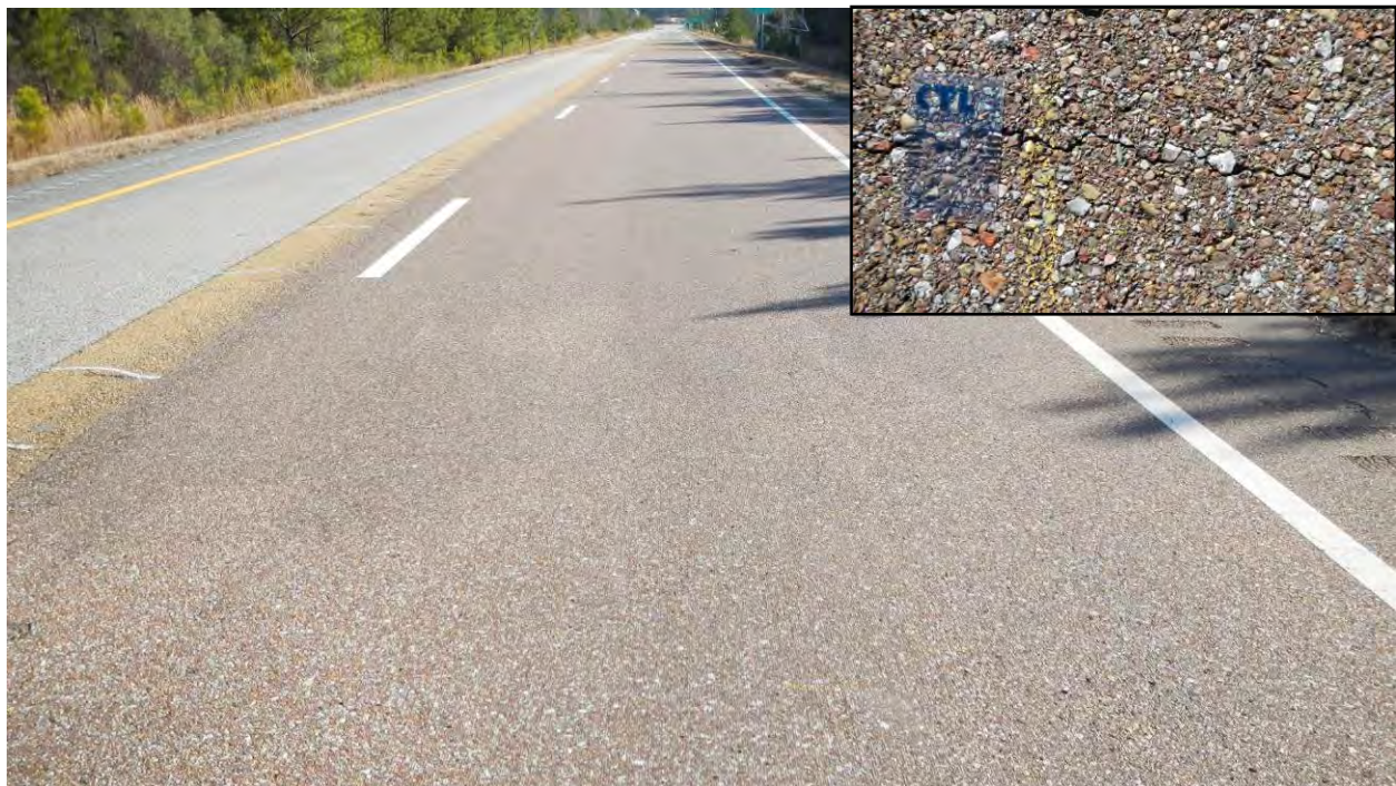
Figure 2.11 Photograph of the MSDOT 45% RAP Test Section after Once Cycle
