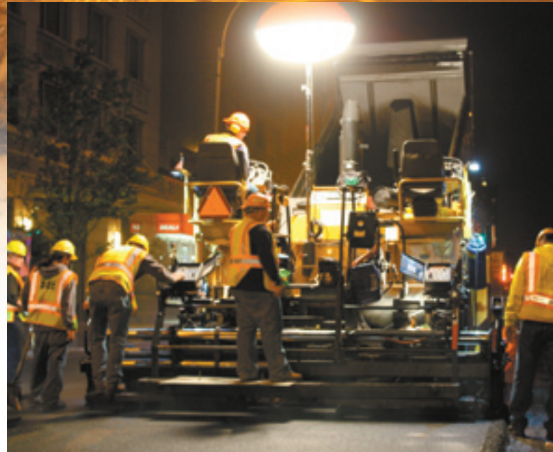
The overlay was applied to a compacted depth of 1-½ inches at the crown, and gradually tapered to one inch at the curbs to maintain curb reveal.
