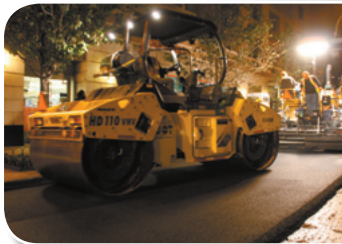
A New York City crew employs a CAT AP1055D Paver and HAMM HD110 Roller during nighttime paving of Manhattan's 1st Avenue with thin HiMA overlay.
