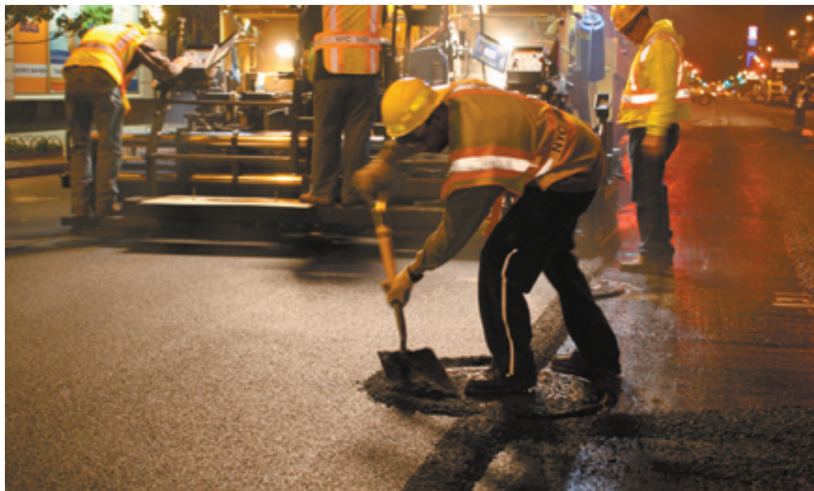
Manhole covers were paved over, then the HiMA modified mix was easily removed from the structures using a shovel.
