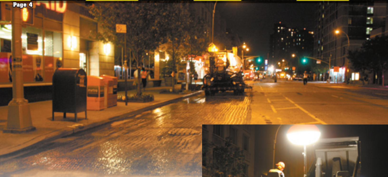
An asphalt distributor truck applies tack coat to the existing pavement before haul trucks begin delivering trial mix to the job site.
