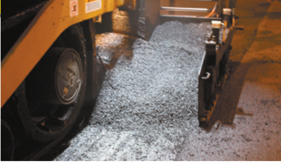
The overlay mixes, which contained 7.2 percent asphalt binder for both HiMA and FlexGard trials, were produced with the plant running normally.
