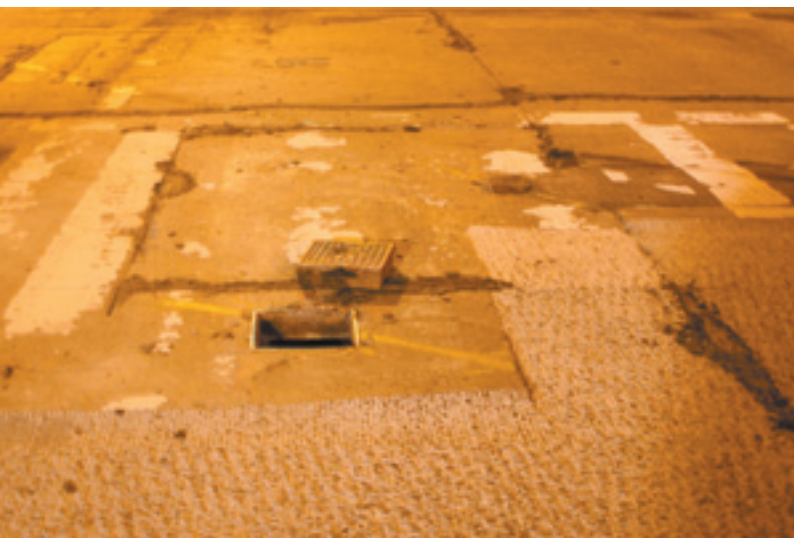
Photo shows milled Portland cement concrete pavement near a manhole of Con Edison, which supplies pressurized steam in 24-inch line to heat buildings.
