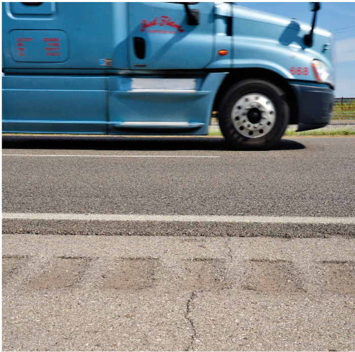
Transverse crack halts at interface with 8-in. HiMA-modified pavement structure.
