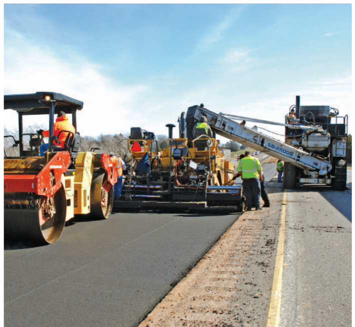
In 2012, material transfer vehicle ensures high quality placement of HiMA modified asphalt lifts.
